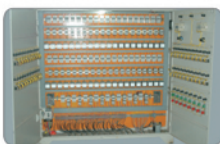
Automatic Raw Cotton Electric Control System Panel
