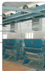
At Site Installed System
